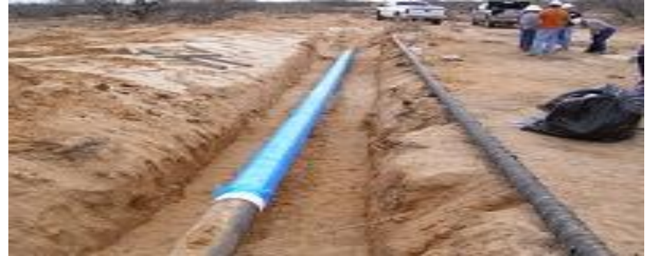
44' linear 10" pipe with 77% external corrosion repaired with wet-layup, in one hour, to reinforce hoop strength. No pressure reduction & backfilled one hour later.
