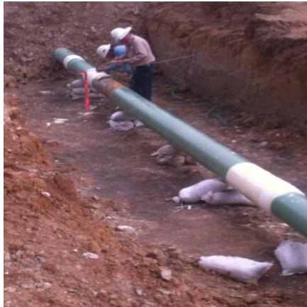
Cigarette wrap isolated external corrosion pitting 68% wall loss.
