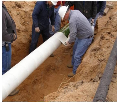
Spiral wrap long sections of external corrosion >80% wall loss. 40 foot joint repair in 1 hr, then back fill 1 hr later.
